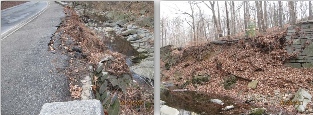
Figure 6. Collapsed Section of Retaining Wall along Piney Branch Parkway Trail
