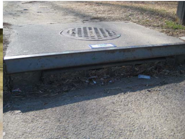
Inlet screens in the Fort Dupont watershed
