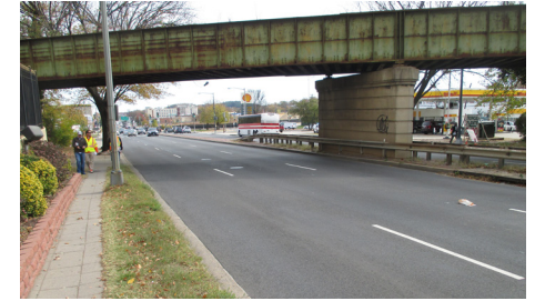
Photo 12: Inactive railroad bridge over New York Avenue NE west of Montana Avenue NE.
